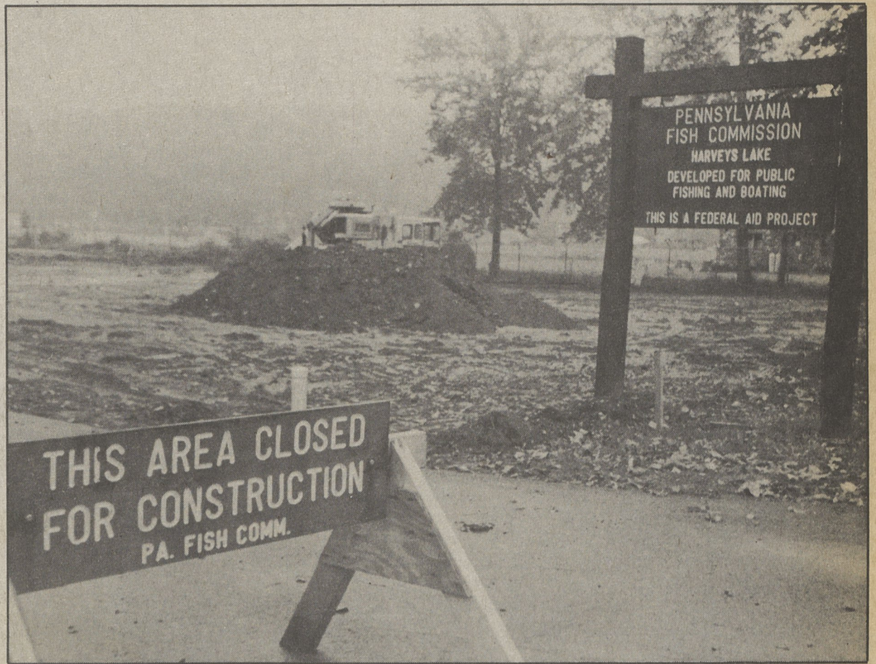
WORK — Signs say the Harveys Lake boat launch will be closed while crews build a restroom and expand the parking lot.
