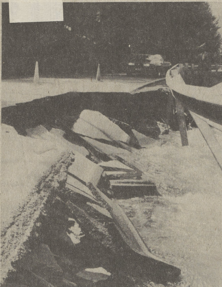
AND THE ROAD CAME TUMBLING DOWN: Literally speaking, it's what happened as heavy spring rainstorms washed out an entire section of Huntsville Road, rendering it impassable. (Dan Walsh Photo)
