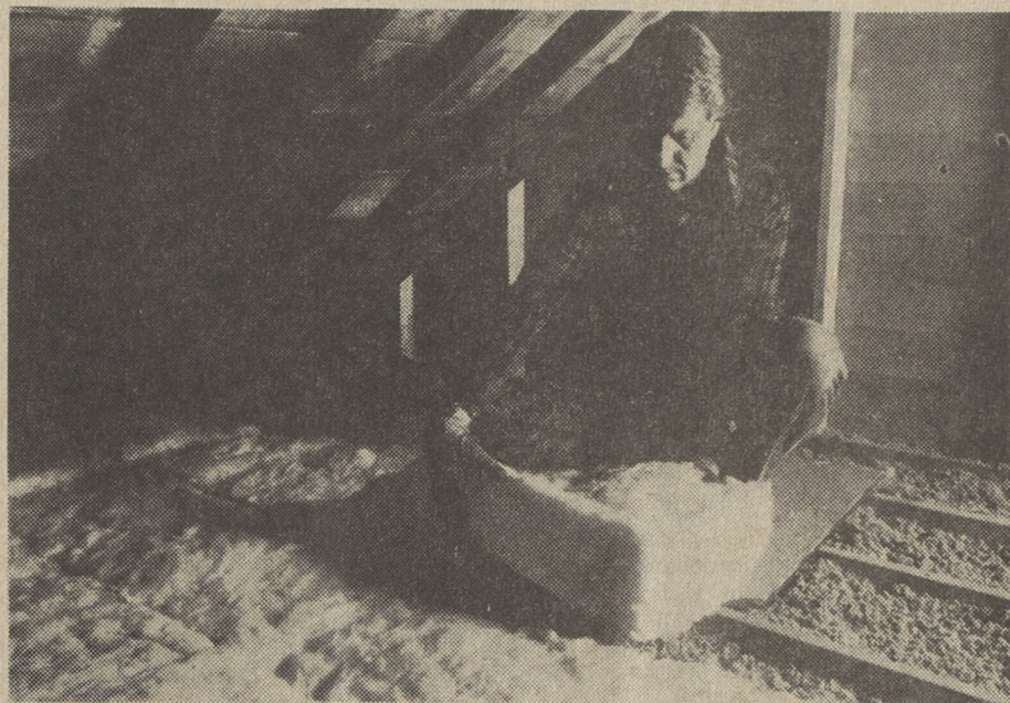
ATTIC INSULATION can substantially reduce the amount of energy needed to air condition and heat the home. Manville's free D-I-Y Home Energy Audit will help you establish your own home energy conservation program.
