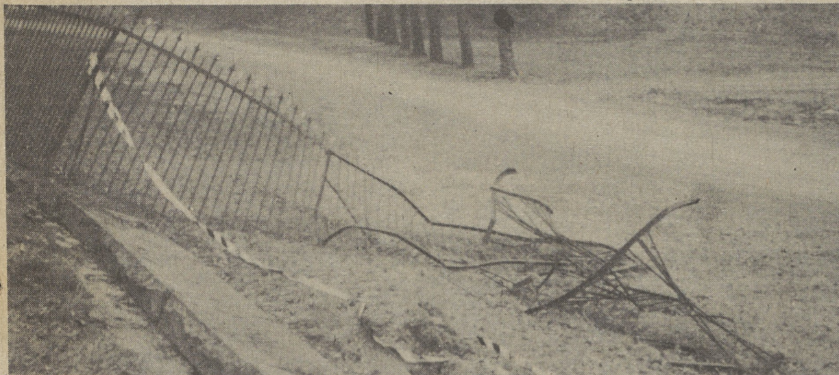
Close to 150 feet of fencing has been ripped down by motorists involved in mishaps near the PG&W Hillside Filter Plant in Kingston Township. The resulting damage is an eyesore, and costly to all drives, since automobile insurance pays for the damage.
