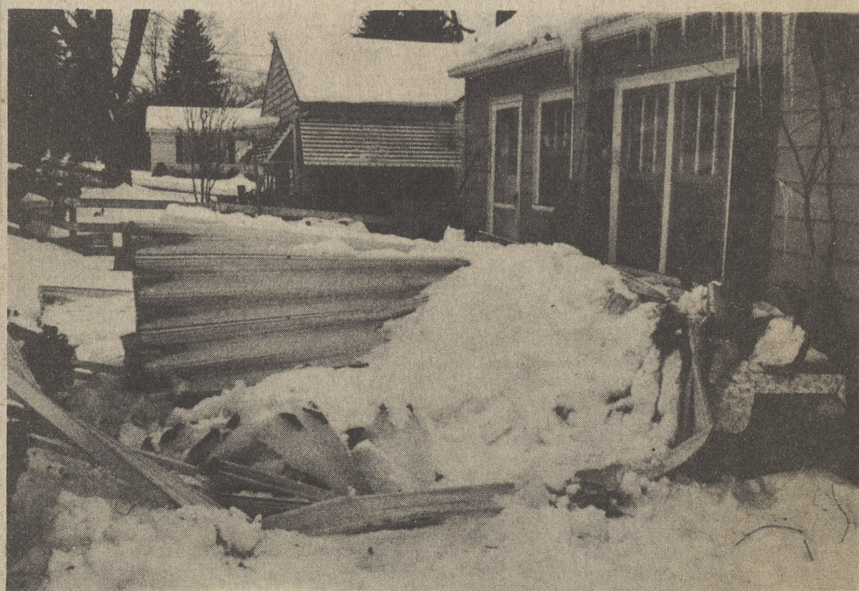
The weight of snow and ice brought down this porch awning at the home of Doris Walters, Terrace Ave., Trucksville.
