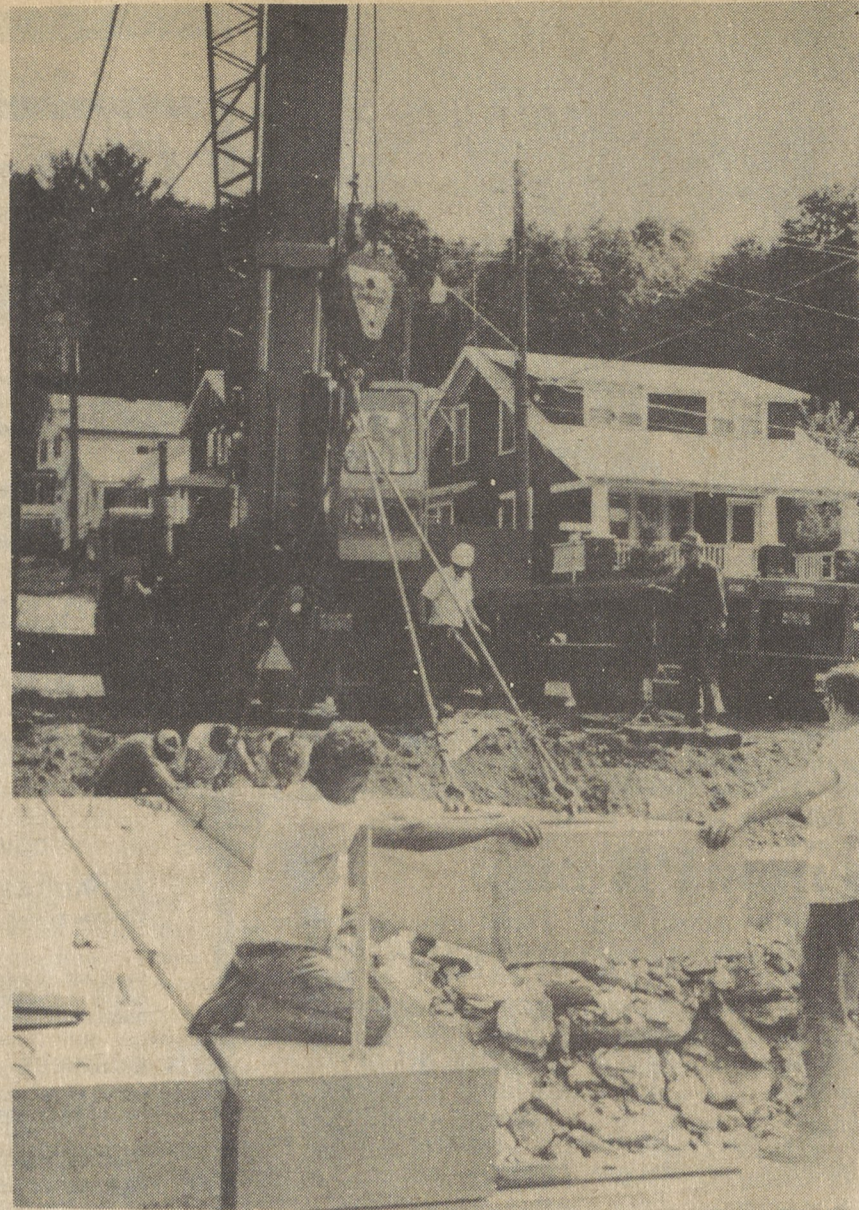
MAKING PROGRESS --Construction workers at the Franklin Street project in Kingston Township guide the first forms for the new bridge which is being built this summer. Work is progressing and the bridge is expected to be completed on time. [Photo by Mark Moran]
