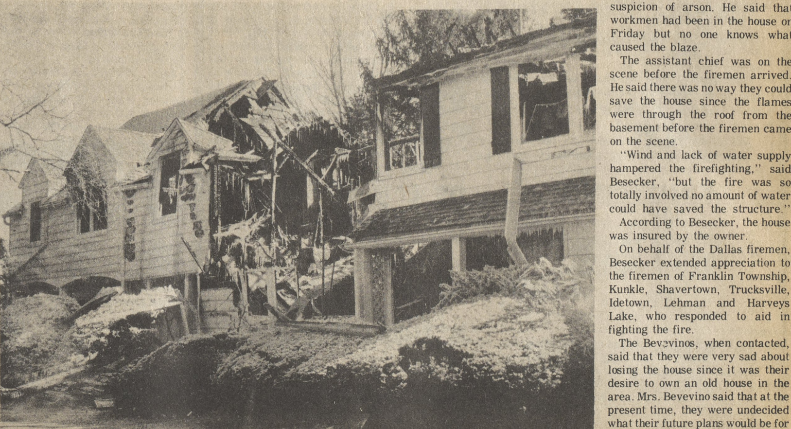
TOTAL LOSS—The large English Tudor home formerly owned by Harrison Smith and recently purchased by Frank Bevevino was totally destroyed by raging flames last Friday night as fireman from six companies were at the scene working to get the blaze under control. (Photo by Mark Moran)
