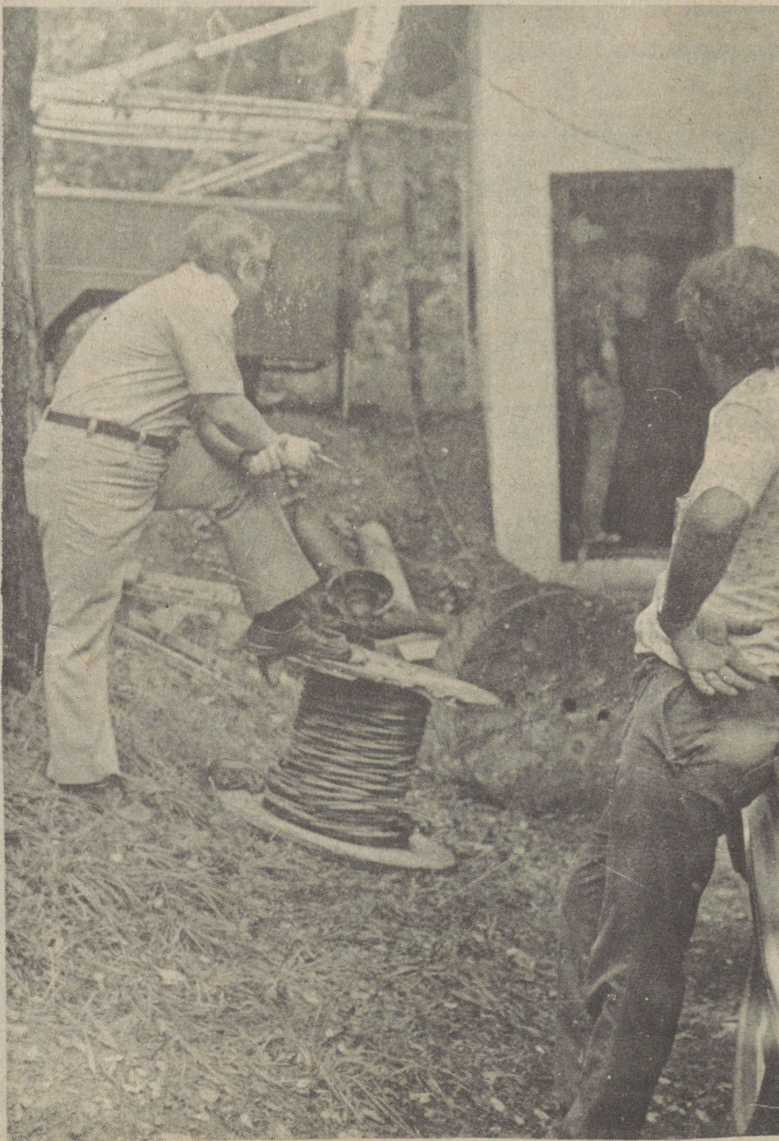
NEW PUMP—Leonard Venable, manager of Dallas-Shavertown Water Company, looks on as employees of Cresswell Drilling Company puts in the pines and installs the new pump at the Country Club Road pumping station. (Photo by Charlot M. Denmon)
