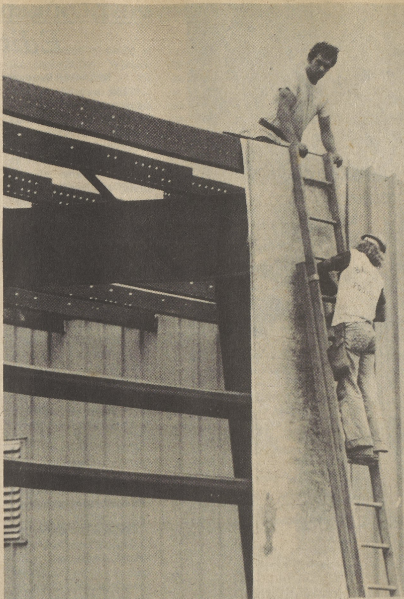
NEW ADDITION--Jack Dieffendorf, at the top, and Mark Shaffer on the ladder, employees of Brandywine Corp., are among the workers aiming to complete the new addition at Energy Convertors, Inc. by the target date of late October. The new addition will have 15,000 square feet of space and provide room for approximately 50 new jobs. (Photo by Charlot M. Denmon)
