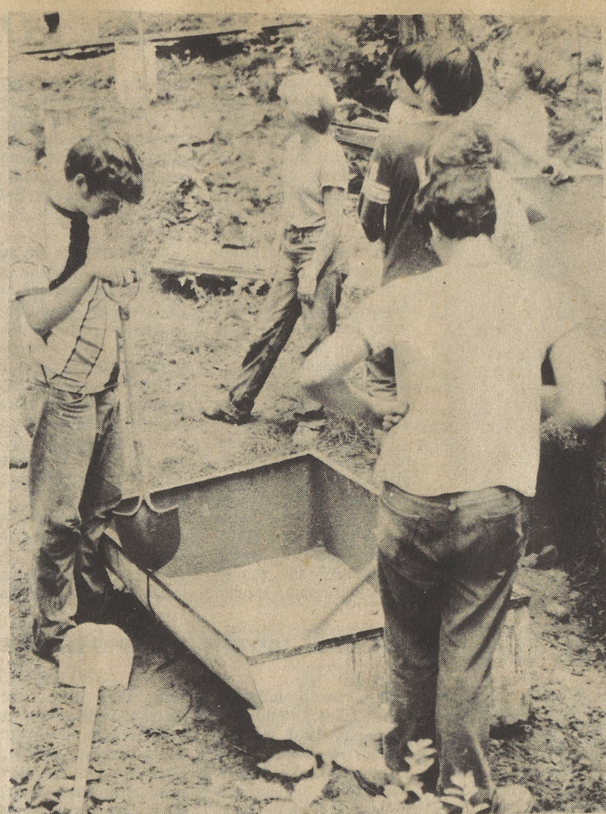
CEMENT MIXERS —These youths from Trinity United Presbyterian Church mix the cement for the supports to the seating for the outdoor chapel at Camp Wilmot, New Hampshire. Left to right are Allan Brague and Dave Brague; in the background are Lori Davidson, Robbie Robinson, Wendy Flick, Scott Davidson and Kim Davidson.
