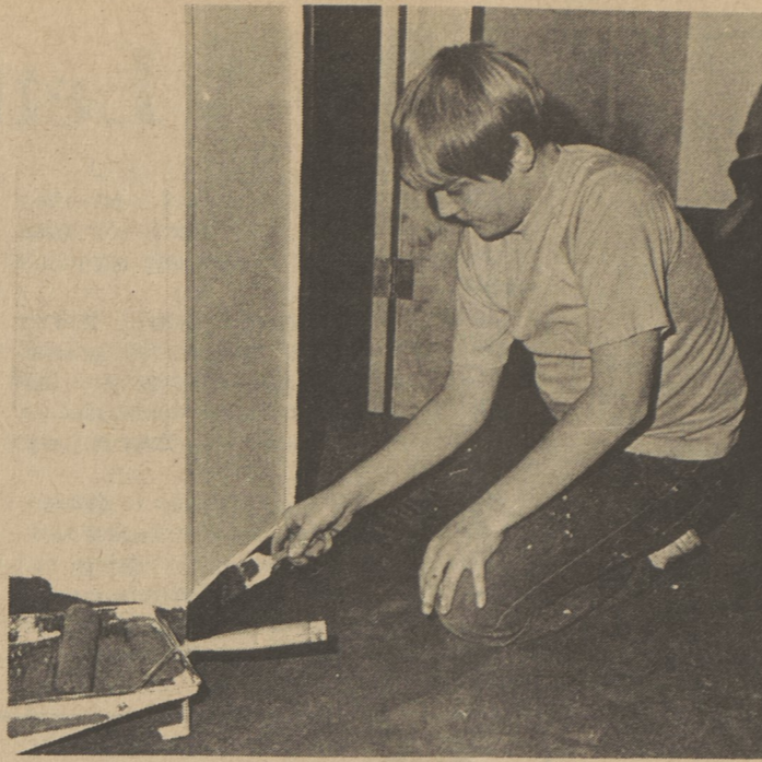
Boy Scout Jeff McDonald of Troop 281 puts finishing touches to his task of painting the basement of Dallas United Methodist Church. This was Jeff's scout community project toward earning an Eagle Badge.
