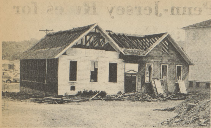
(J. KOZEMCHAK SR.) One of the oldest educational landmarks in Dallas School District is being razed. Shavertown Elementary School Annex was built in 1924, and the one-story wooden structure has housed several generations of students.
