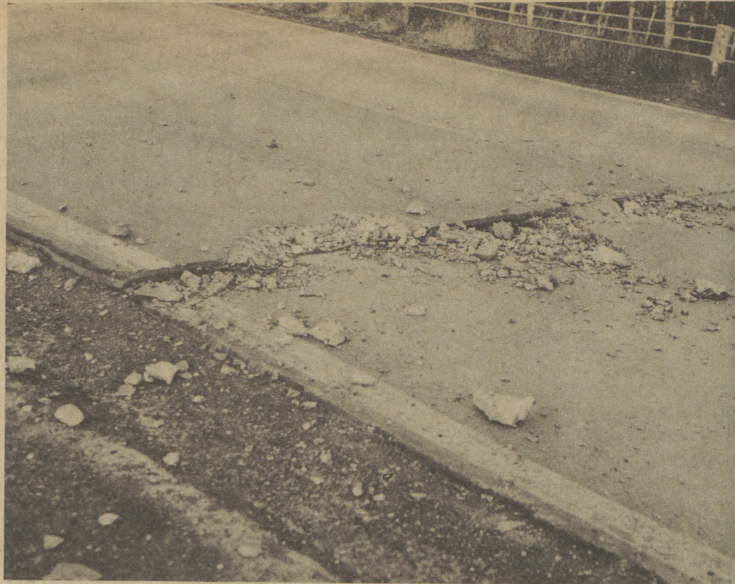
A sharp rise in temperature Monday about mid-afternoon caused an explosion between two concrete sections of Route 118, going west toward Lehman Center. Residents in the immediate area heard the loud report and find large pieces of concrete blown as far as 15 feet away. Lehman Township officials said the explosion was the result of expansion, due to heat. The highway is maintained by the State Department of Transportation, whose area representative said he did not know when the pavement would be repaired.
