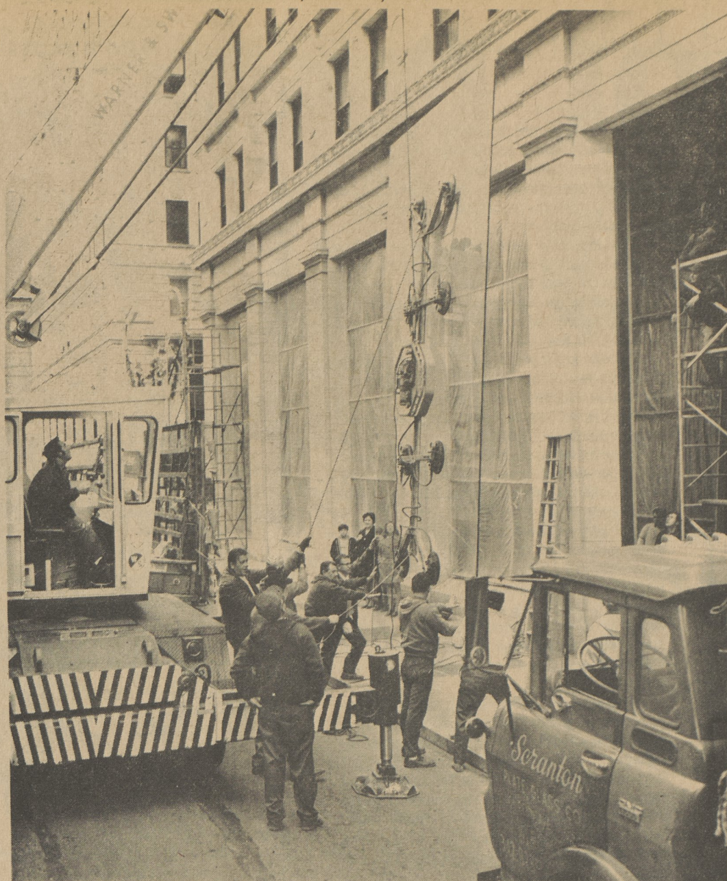
Raymond R. Hedden Company, Dallas, steadies the largest plate glass window in the region as it is positioned into the framework at the United Penn Bank, Wilkes-Barre.
