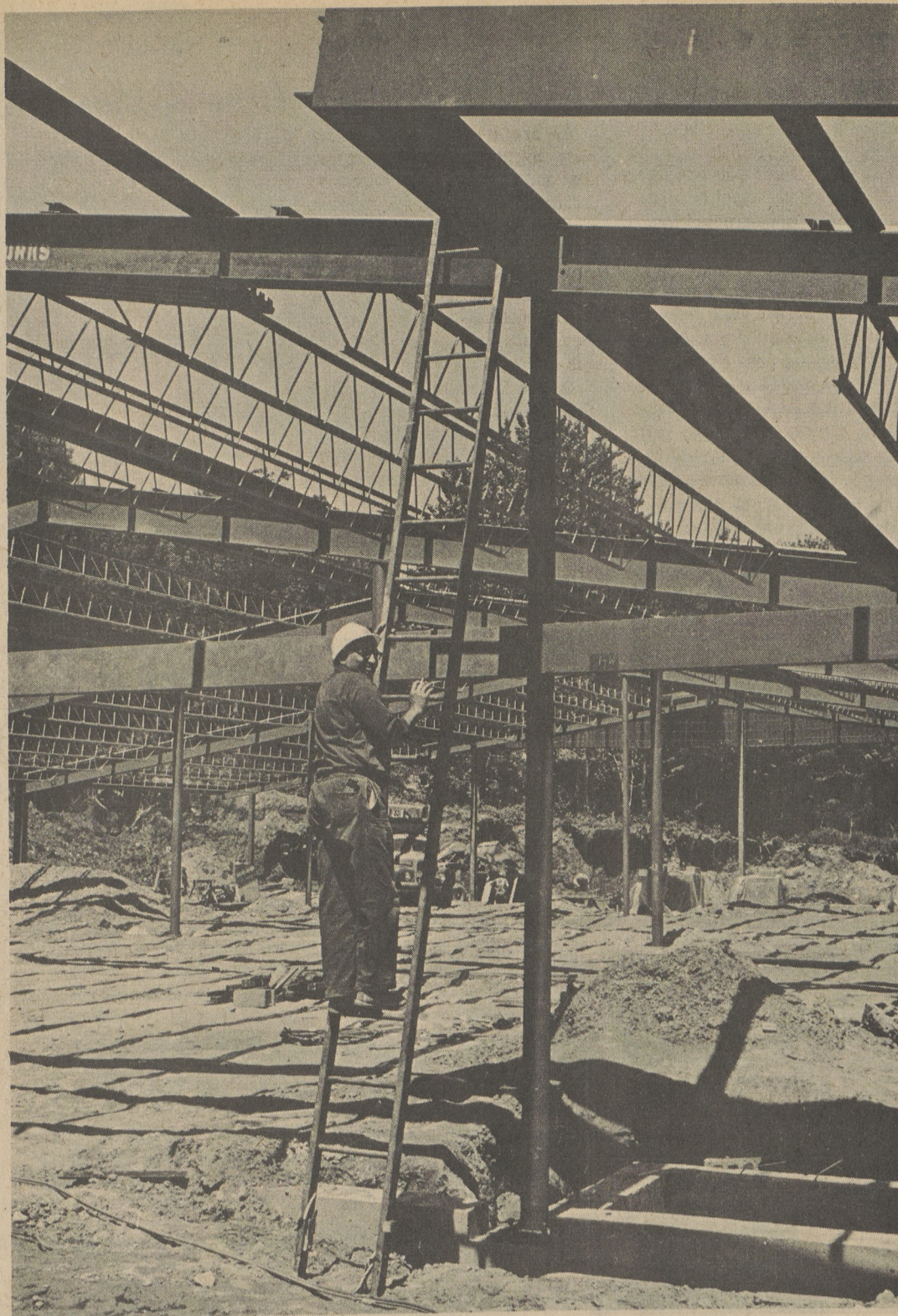
Worker climbs ladder at construction site of new Dallas Acme market. Steel work went up last week.
