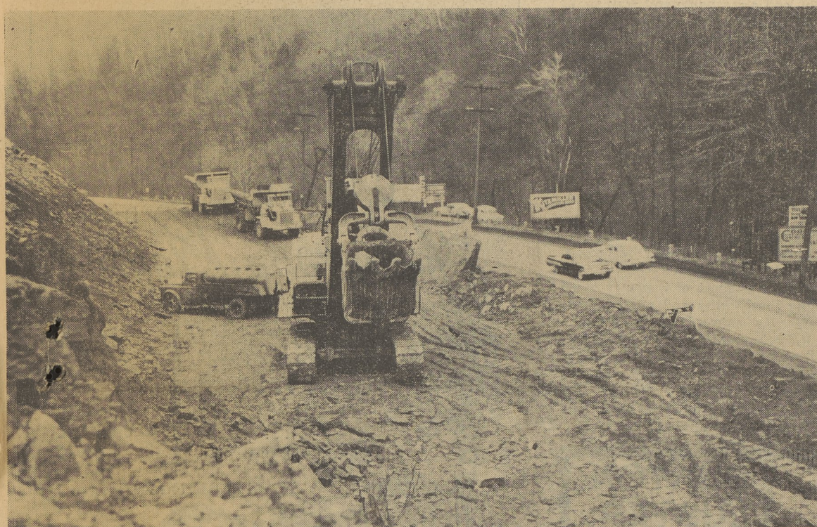
TWISTING HIGHWAY , between the "big bend" and Hillside road, was straightened out some, as part of the new highway work completed this year. Picture shows shovel chewing away the mountainside in April. Highway was dedicated in October.
