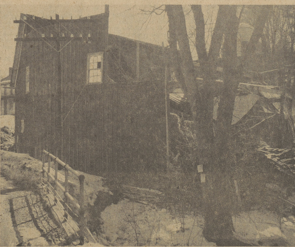
This is what is left of Ray Prutzman's Barn, a familiar landmark on the Hillside-Huntsville Road, after heavy snows crushed the already aging structure. Fortunately the herd of cows in another part of the structure was unmolested although damage to the section devoted to storage was considerable. —Photo by Kozemchik
