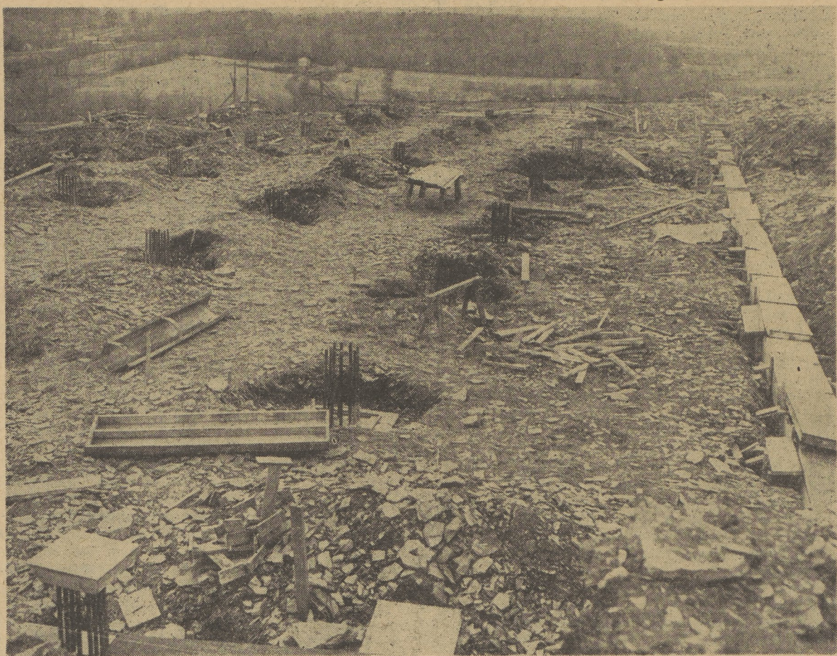
Forms are poured for the first building—a warehouse—that will be erected at the new State institution for Mental Delinquents in Jackson Township. The building is located high above the surrounding countryside. Actual construction is not expected until March after all blasting and rough grading is completed. —Photo by Kozemchak
