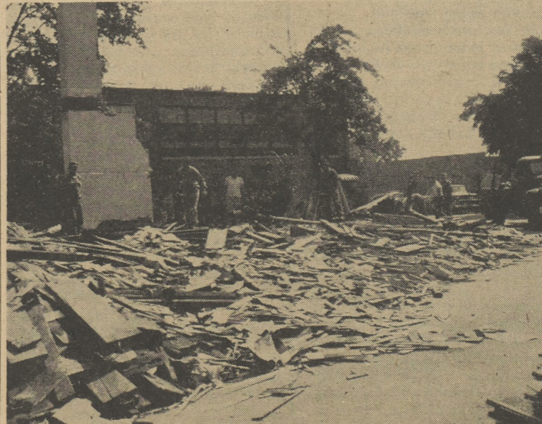
This stark chimney and pile of rubble is all that remains of the former Bauer home, Machell Avenue and Spring Street, which is being torn down by contractor John Parrish to make way for the new addition to Gate of Heaven School. Work of razing the building started a week ago Monday and was completed in eight days, twelve days ahead of schedule.
