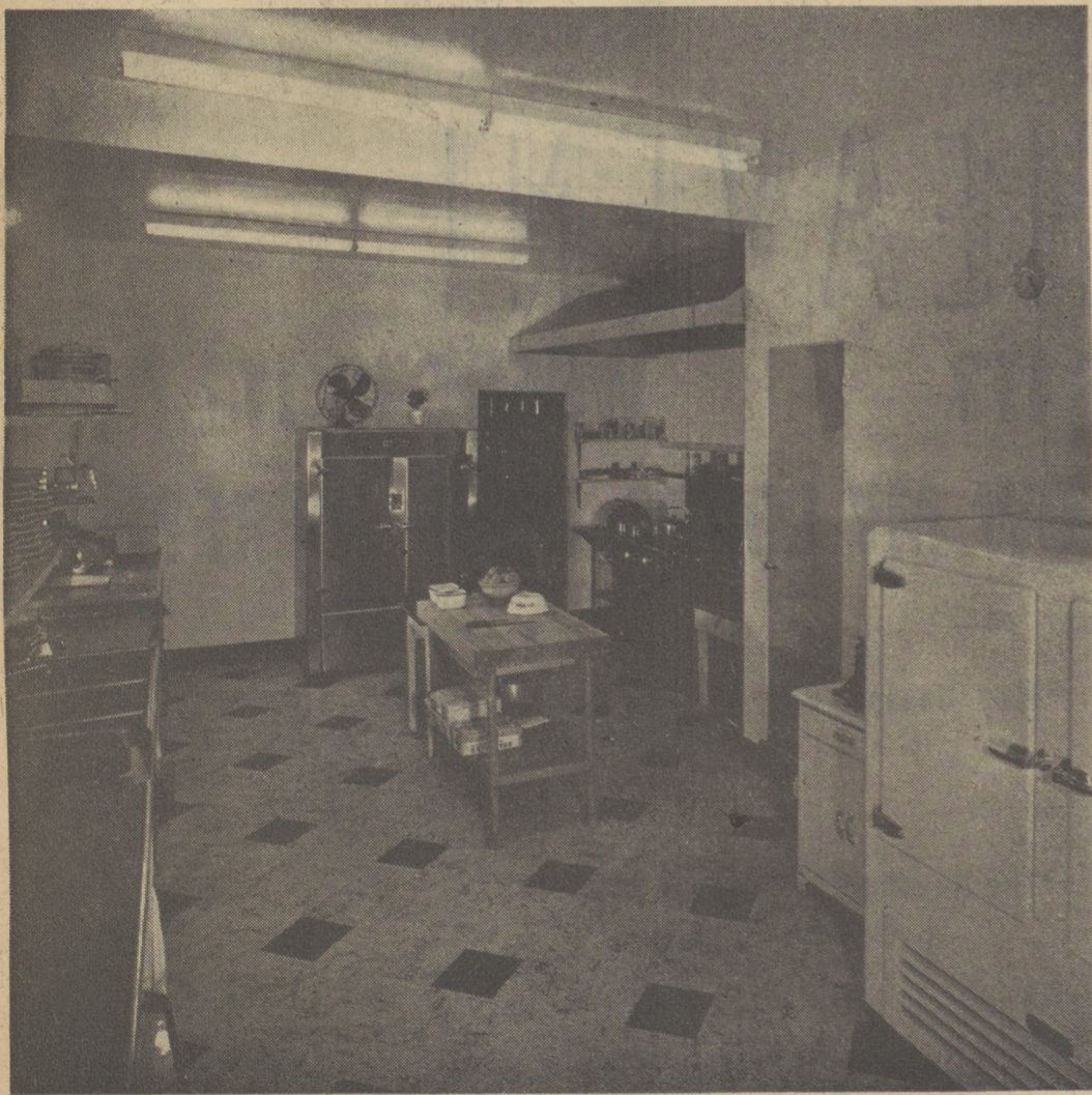
A part of the spic and span, daylight kitchen equipped with the most modern gas and electric cooking and refrigeration equipment for preparing and serving delicious food.
