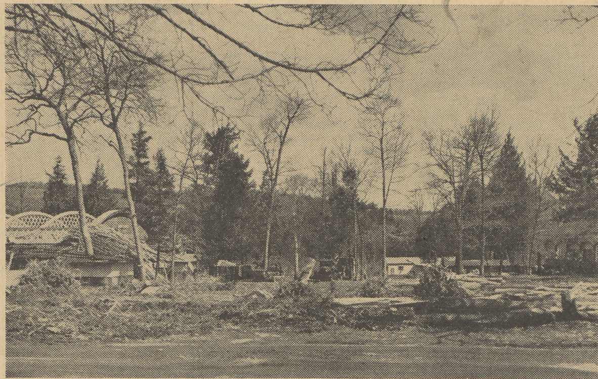
Fernbrook Park takes on an unfamiliar aspect as woodsmen fell trees and wrecking crews raze buildings to clear the ground for the new plant of Bloomsburg Mills.
