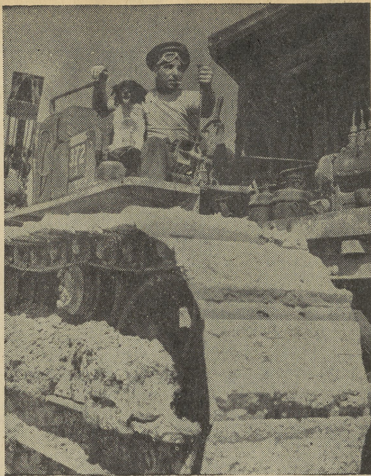
"Babe" Thompson of North Bay, Ontario, with his dog, "Butch," perched beside him, drives an American tractor as he works on construction of a new road in Britain. Canadian roadmakers in England are being kept busy carving out new military highways and repairing old roads blasted in air raids. (Central Press)
