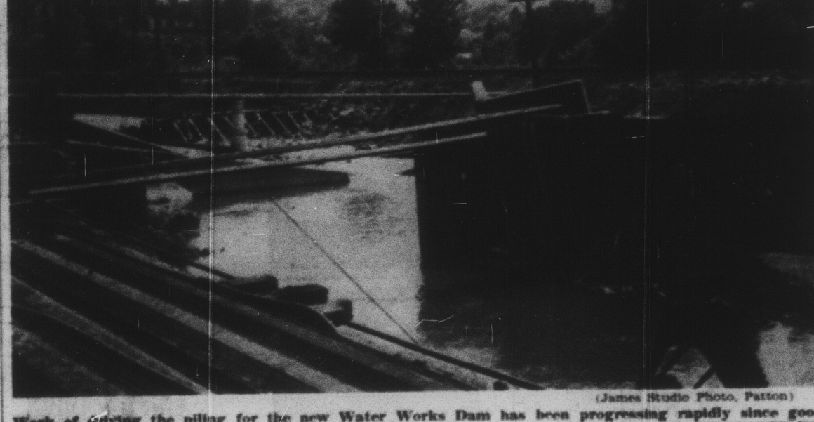
Work of driving the piling for the new Water Works Dam has been progressing rapidly since good weather set in. The dam replaces one washed out a year and a half ago. Since that time water has been diverted into the pumping station by means of a temporary breastwork shown in the upper left of the picture. Patton residents use an average of 500,000 gallons of water per day.
