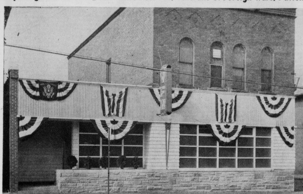
Work is nearly completed on the construction of a new building and the remodeling of the old structure of John White Post 779, VFW, Patton. A grand opening is planned in the near future, according to post officials. The post was founded in 1934 and named after John White, a World War I veteran, son of the late James and Mrs. Rebecca White of Patton. It now boasts a total of 421 regular members and 400 associate members. Work on the project was begun last December by George C. Hoppel. (Photo by James)
