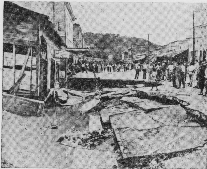
Undermined by flood waters from a swollen tributary of the Alabama river, this section of the Prattville, Ala., main street collapsed, halting traffic through the business district. Floods were caused by heavy rains, and though there was no loss of life, more than 3,000 persons in the southern part of the state were forced to flee their homes.
