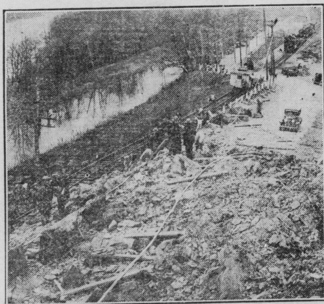
When workmen engaged in a construction project along the Reading-Pottsville Pike set off an unusually heavy charge of dynamite recently, the roadway was buried beneath 150 tons of earth and rock. The Reading-Wilkes-Barre cable of the Bell Telephone Company was torn from the poles and covered by the debris. While emergency crews were rushing repairs, telephone calls were being routed over other lines.
