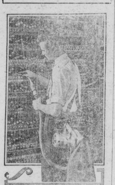
A Bell Telephone maintenance man shown using a vacuum cleaner to remove dust from the mechanism in a "dial" telephone exchange.
