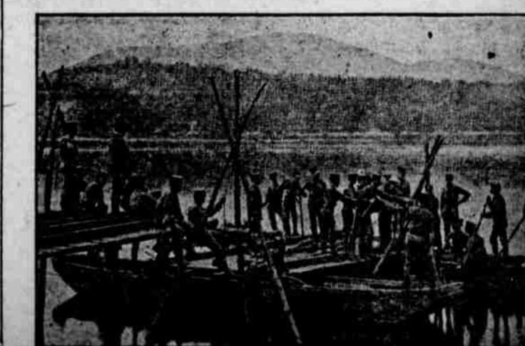
Building a Trestle Bridge at the United States Military Academy at West Point
