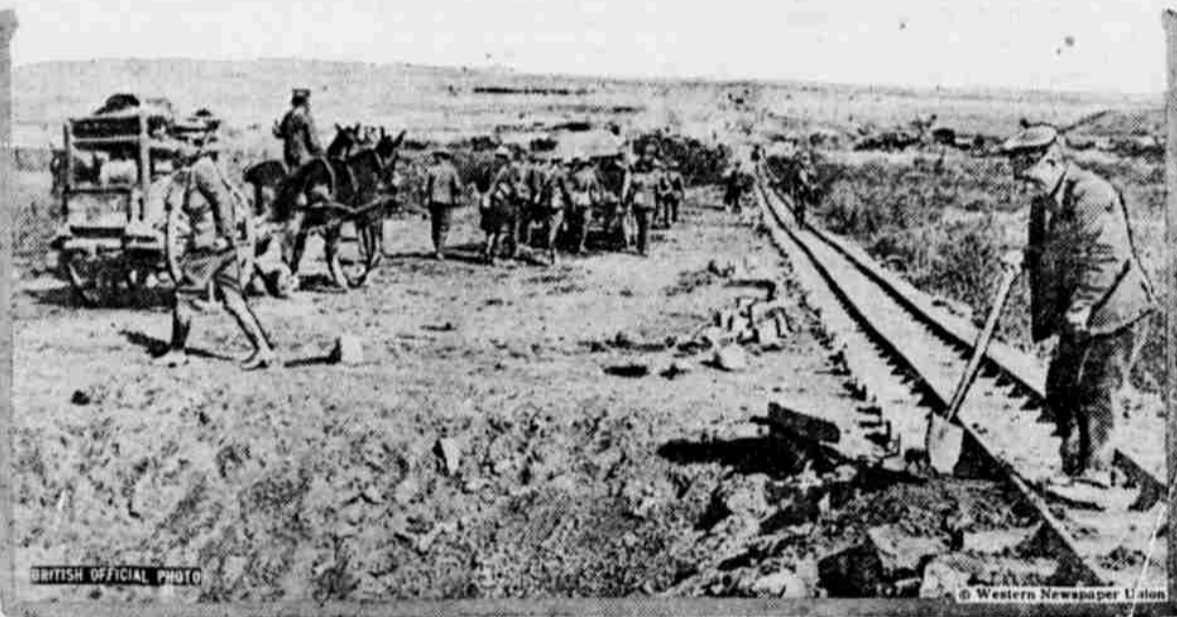
The reconstruction period is now sweeping over all of the battle-scarred area of France and the roads are being rebuilt. This photograph shows a scene on a road in the vicinity of Cambrai that was mined by the retreating Germans. The British constructed a light railway and a new road.
