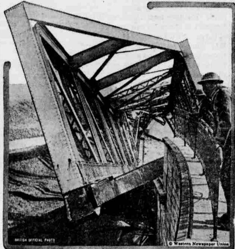
Bridge across a canal destroyed by the Germans in the retreat in northern France.
