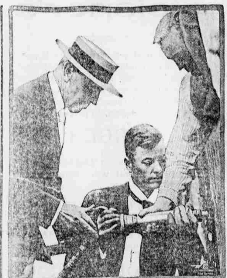
President Wilson is here seen driving the first rivet in the keel of a 10,000-ton cargo carrier, this being the first keel to be laid in the steel shipyards at Alexandria, Va.
