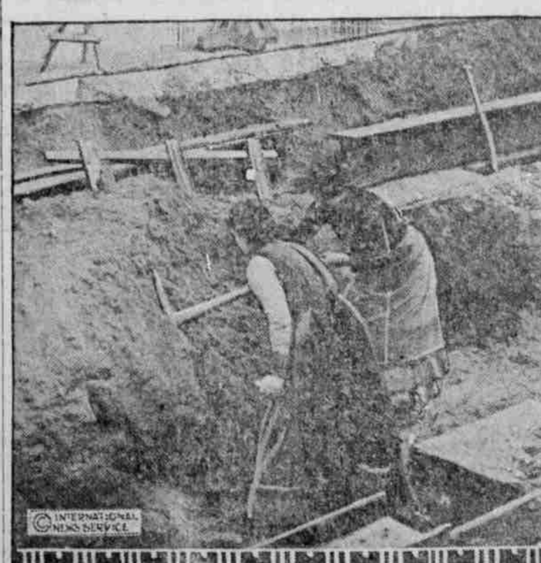
The fact that the menfolk of the German capital are on the various battle fronts does not in any way hold up the civic improvements of Berlin. The construction of the Berlin subways is being carried on mainly by women. They are doing nearly all the work that was formerly done by men and are doing it well.
