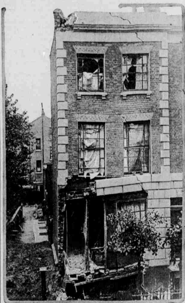
What the bombs dropped from the German Zeppelins in their recent raids over London did to the buildings where they fell is well illustrated by this photograph of a house in Shakespeare road, badly wrecked and seemingly about to collapse.
