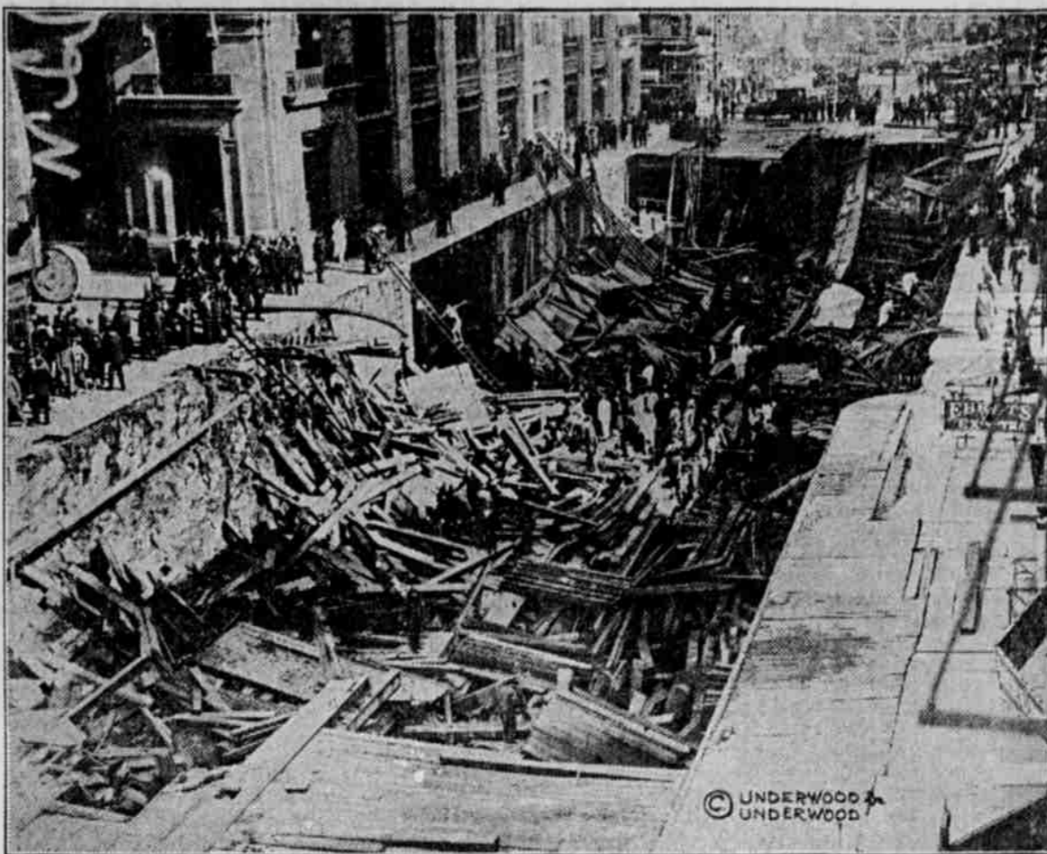
As a result of a blast of dynamite in the new subway under Seventh avenue in New York, an entire block of that thoroughfare, from Twenty-fourth to Twenty-fifth street, collapsed. A crowded street car dropped into the chasm. Seven persons were killed and nearly a hundred injured.
