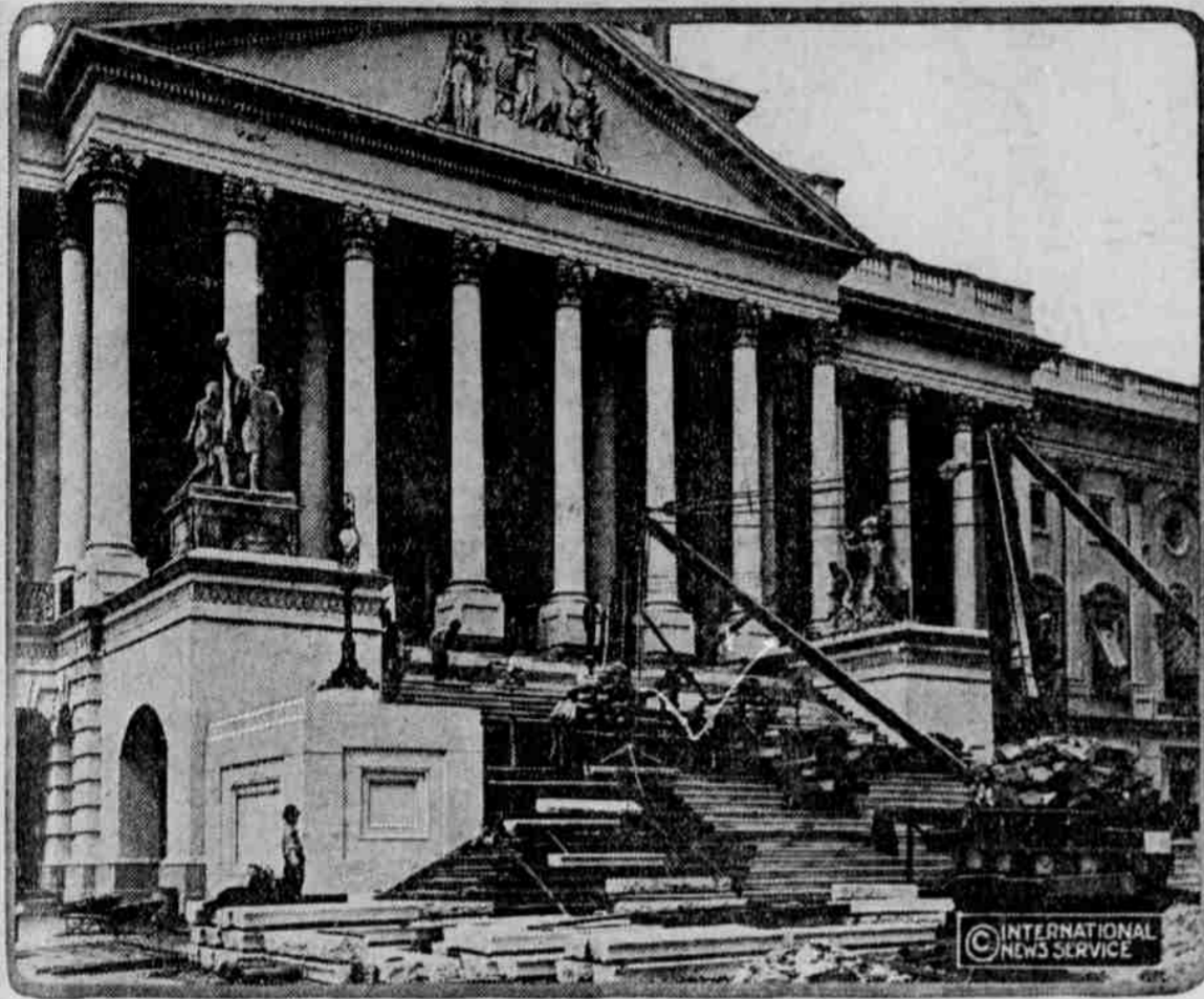
Workmen putting in new marble steps at the capitol at Washington to replace the old sandstone steps which time and the weather had rendered unsightly.
