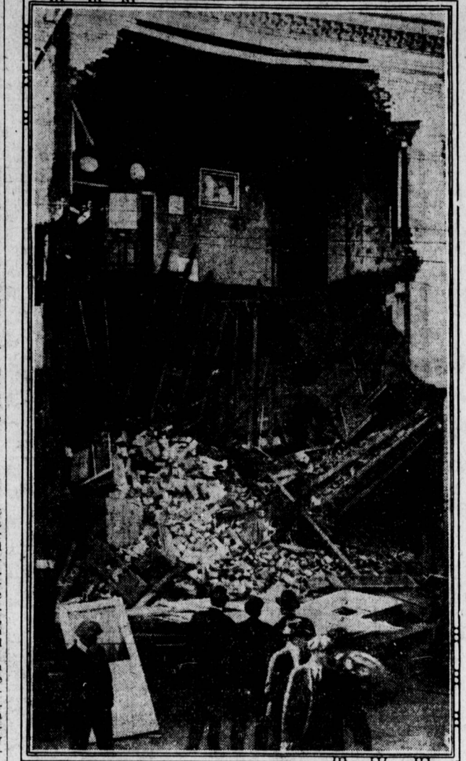
Frederick, Md., April 19.—Many narrow escapes were made when the entire front wall of the Byerly building toppled into the street. A number of men were busy at remodeling operations, and, although the wall collapsed without warning, not one of them was injured. The other walls and the interior remained intact, as can be seen by the pictures hanging on the walls in the above illustration. Several persons in the street narrowly escaped injury.
