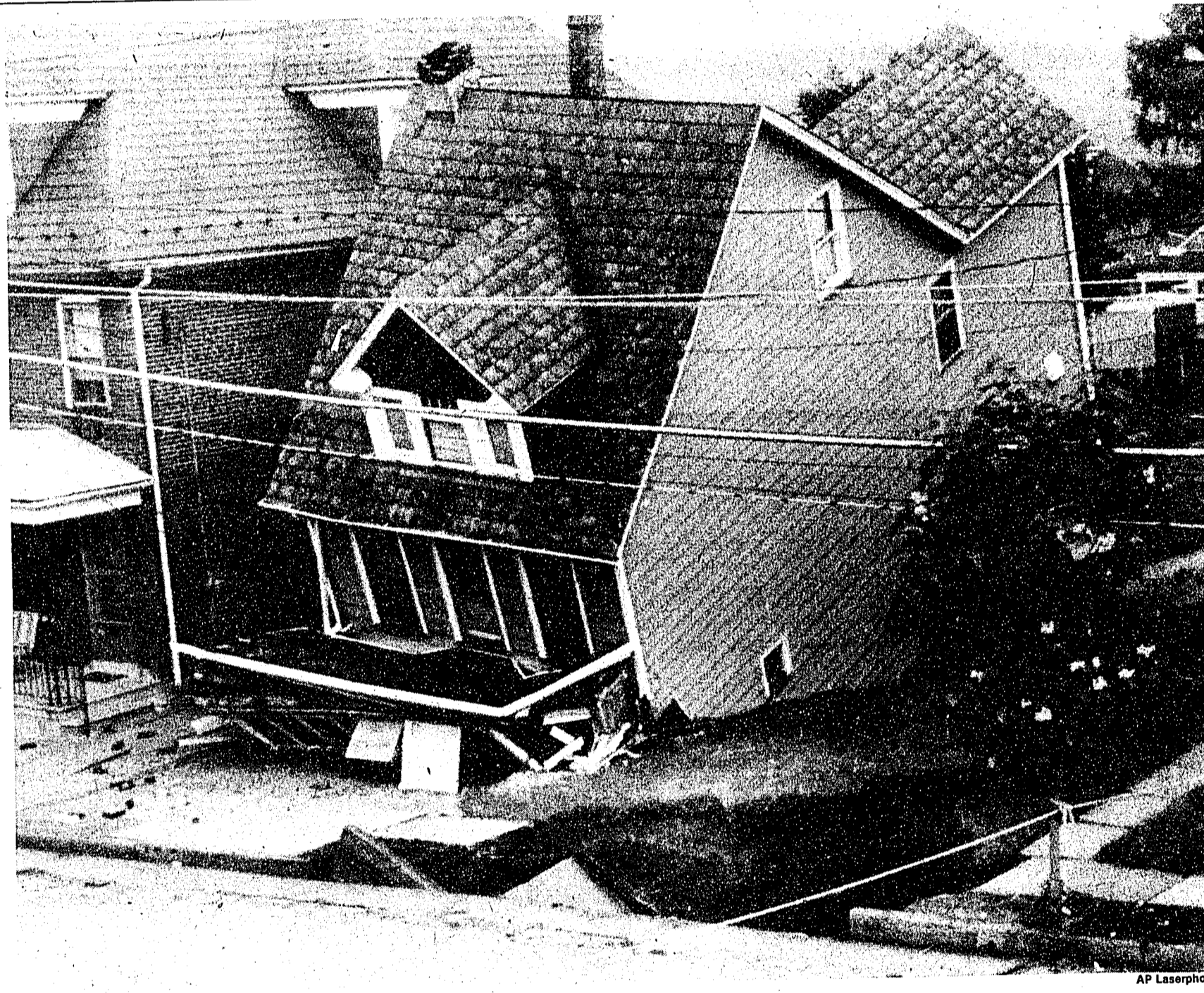
Fallen tavern Dot and Shorty Vosseler's tavern on Thomas Street in Phillipsburg, N.J., collapsed yesterday when the second story of the tavern sank to ground level after water from a broken pipe washed away the earth supporting the building. With the help of police, those in the building fled without injury.
