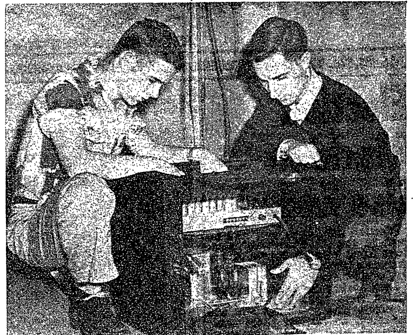
WDFM ENGINEERS David Richardson, left, and Phillip Scott, right, make adjustments on the transponder installed in the basement of Hamilton Hall. The transponder receives FM waves from the station and converts them to AM waves which are transmitted over dormitory power lines. The transponder serves the entire West Dorm area, including Hamilton, Thompson, McKee, Irving, Watts, and Jordan Halls.
