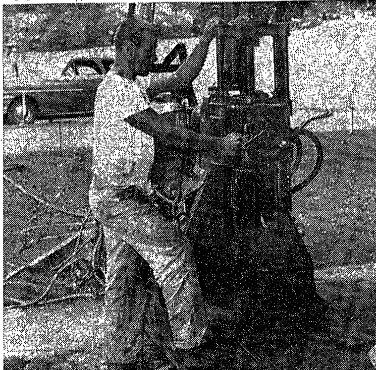
DRILLING RIGS on Holmes field this week caused discussion among students about the proposed Student Union building. College officials however said that the building was no closer to completion than previously since the tests were being taken only as a means of discovering what problems would be met if the building were started.
