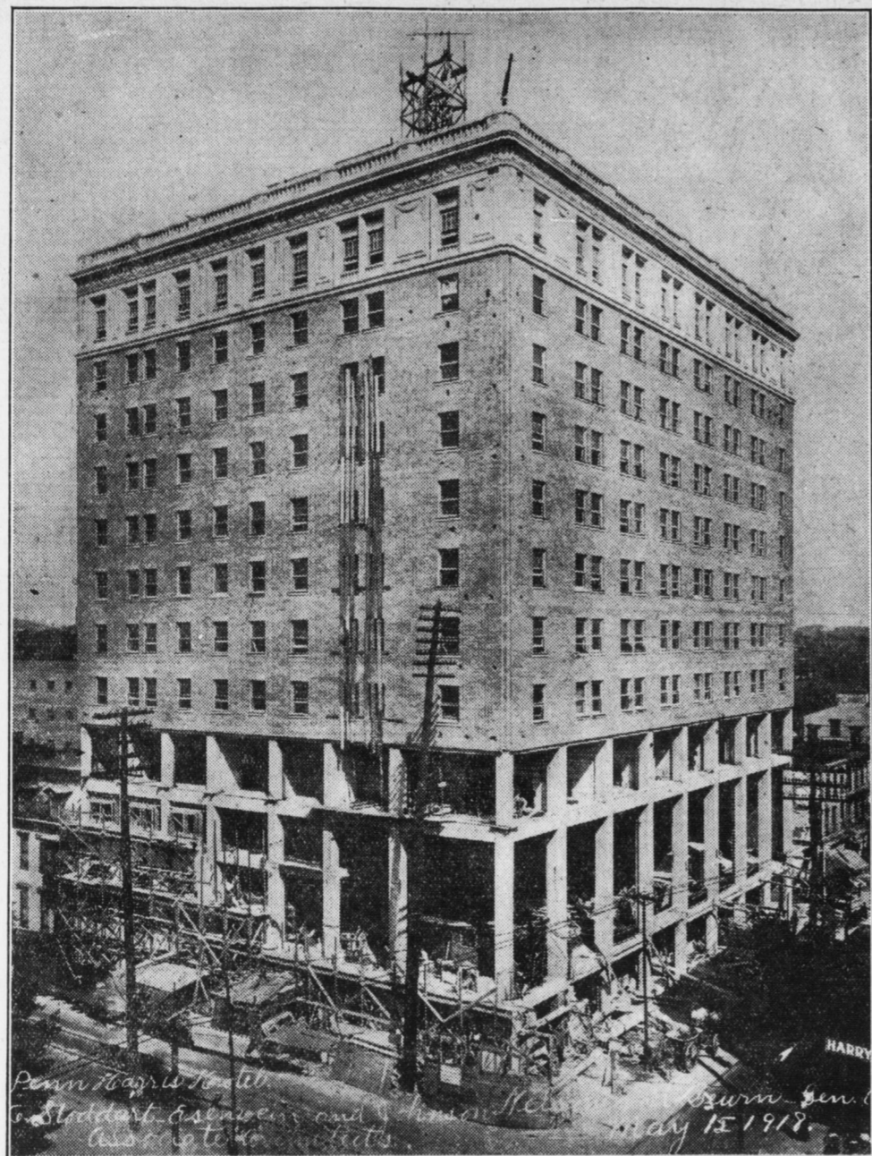
The photograph shows the new million-dollar Penn-Harris hotel, which is almost completed. The ornamental cornice just below the roof has been finished and there are but a few floors to be finished with the exterior brickwork. The building will be turned over to the upholsterers and interior decorators in a short time.
