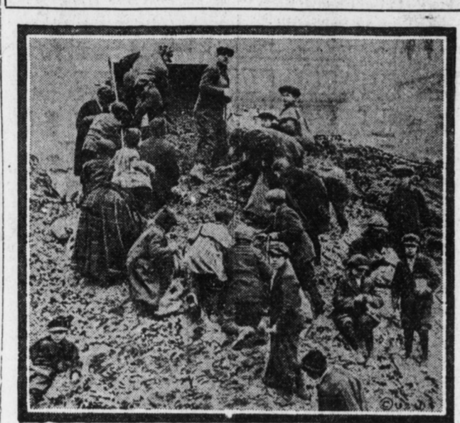
From the many municipal buildings in New York city some hundreds of tons of ashes are dumped every day on the site to be occupied by a new and costly county courthouse. Each morning hundreds of men, women and children from the nearby tenements scrape over the ashes to pick the lumps of coal that slipped through the furnace grates. Tons of coal are thus carried off each day to warm tenement dwellers who might otherwise suffer.
