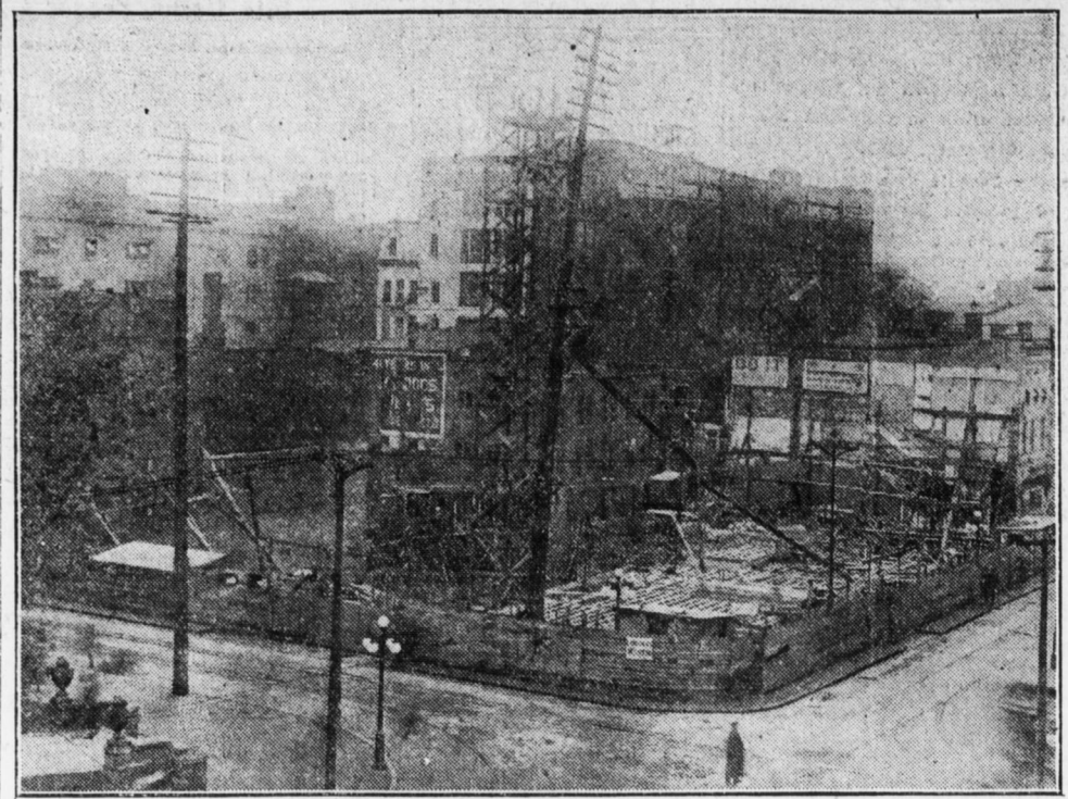
The above etching shows the progress made on the new Penn-Harris Hotel at Third and Walnut streets. The excavation work has all been completed and concrete is now being poured into the foundations. It is expected to have the hotel under roof before next Christmas.
