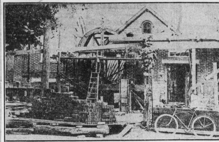
Construction of a new church building in Carlisle, Pa., showing the old structure being incorporated into the new design.
