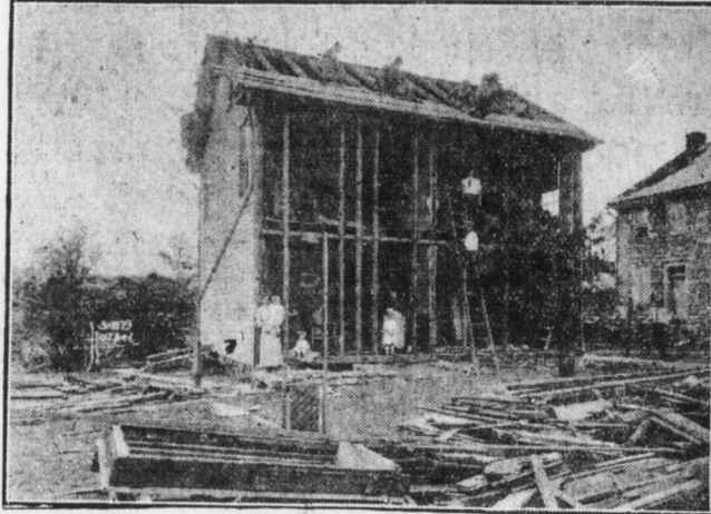
SIDE OF HOUSE BLOWN OFF. The home of Zacharias Bowman, postmaster of Anncville for many years, was wrecked in the way that the etching above shows. The side of the dwelling was completely ripped off by the cyclonic winds.
