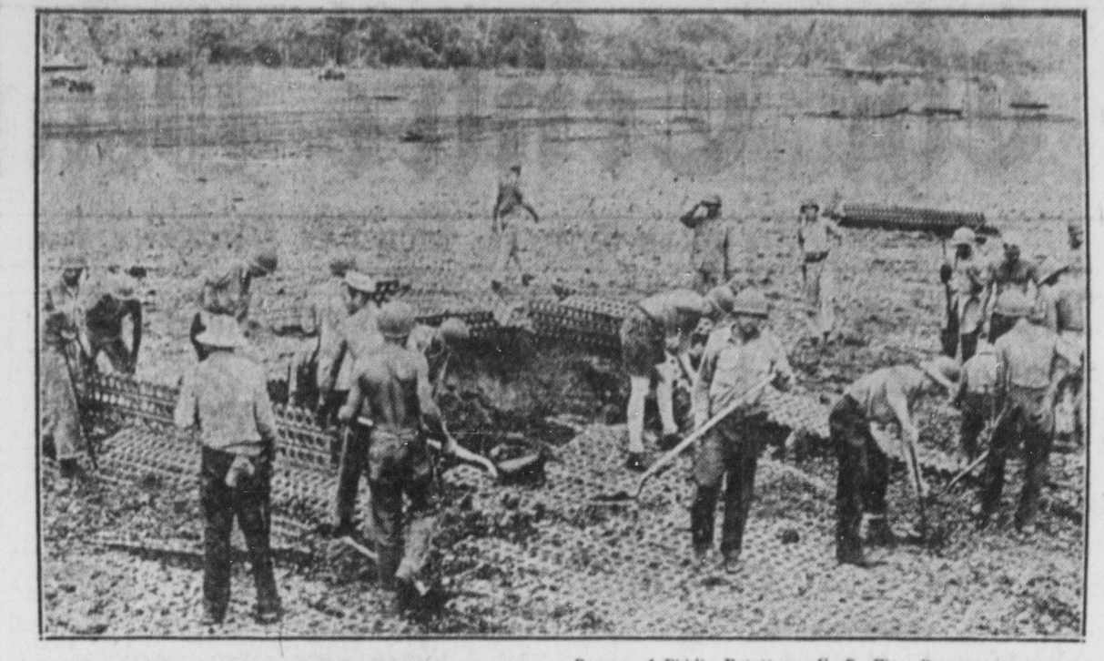
Bureau of Public Relations, U. S. War Department LIGHTNING REPAIRS OF BOMB DAMAGE—Sometimes it is merely a matter of minutes after enemy aircraft bomb an airfield until U. S. Army Aviation Engineers are on the job repairing the damage.
