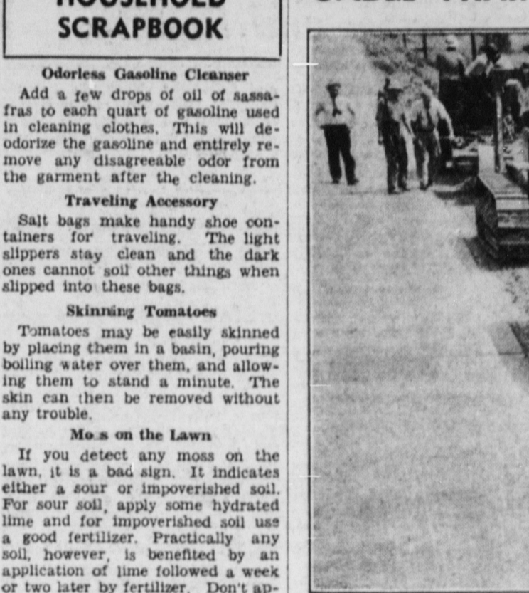
The Bell Telephone Company's "cable train," as it appeared in use for the first time in Central Pennsylvania, along highway route No. 64, ten miles east of Bellefonte. The three-tractor train digs a 30-inch furrow, lays telephone cable in it and covers the cable with earth—a complete job all in a single operation.
