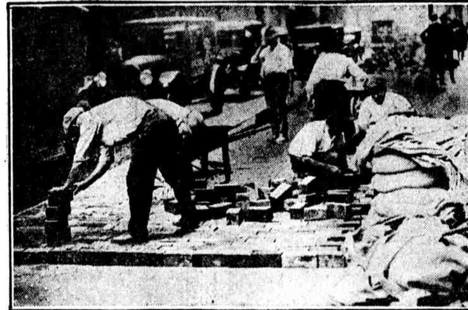
REPAVING CHESTNUT STREET. At Thirteenth street the Chestnut street conduits of the Western Union Telegraph Company have been placed and covered over. The paving blocks are being set in place
