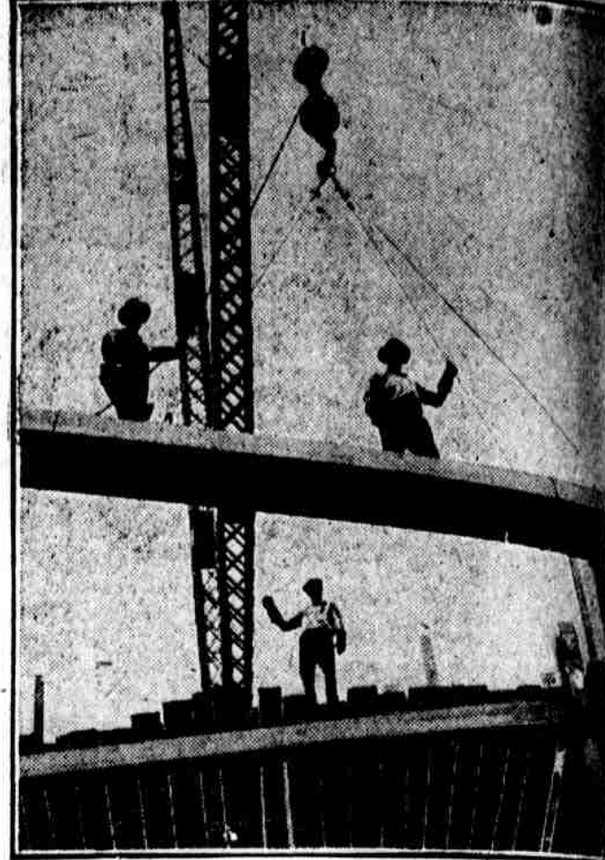
A SILHOUETTE. Observers are amazed at the rapidity with which the office building at Seventh and Chestnut streets is being erected
