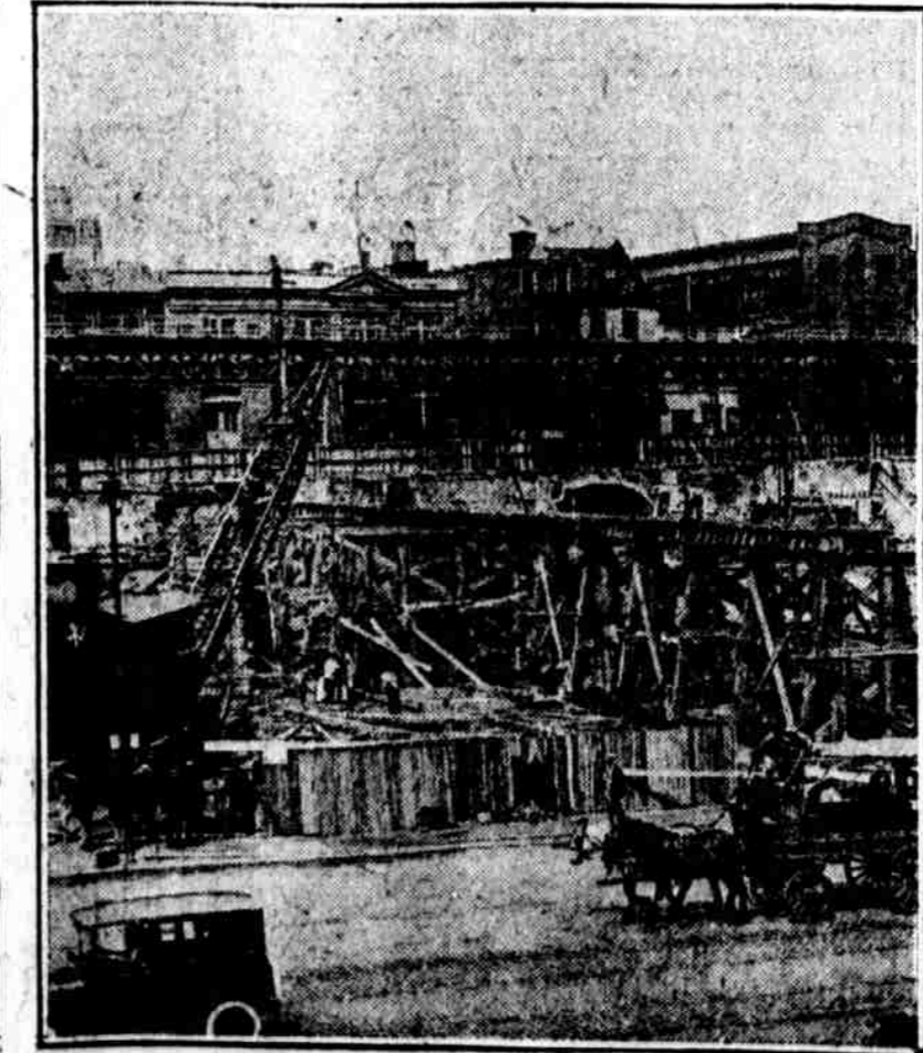
BUILDING A RAILROAD TO THE PHILADELPHIA CAISSON. By this means material will be carried over Delaware avenue. Two new steam shovels have arrived to be used in excavation work
