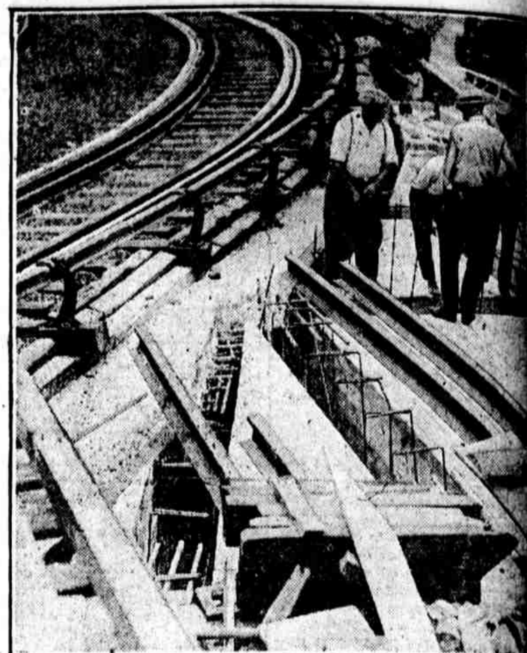
GETS CLOSER EVERY DAY. There is very little space left between the structure of the Market street "L" and the tracks of the Frankford "L." They'll soon be connected
