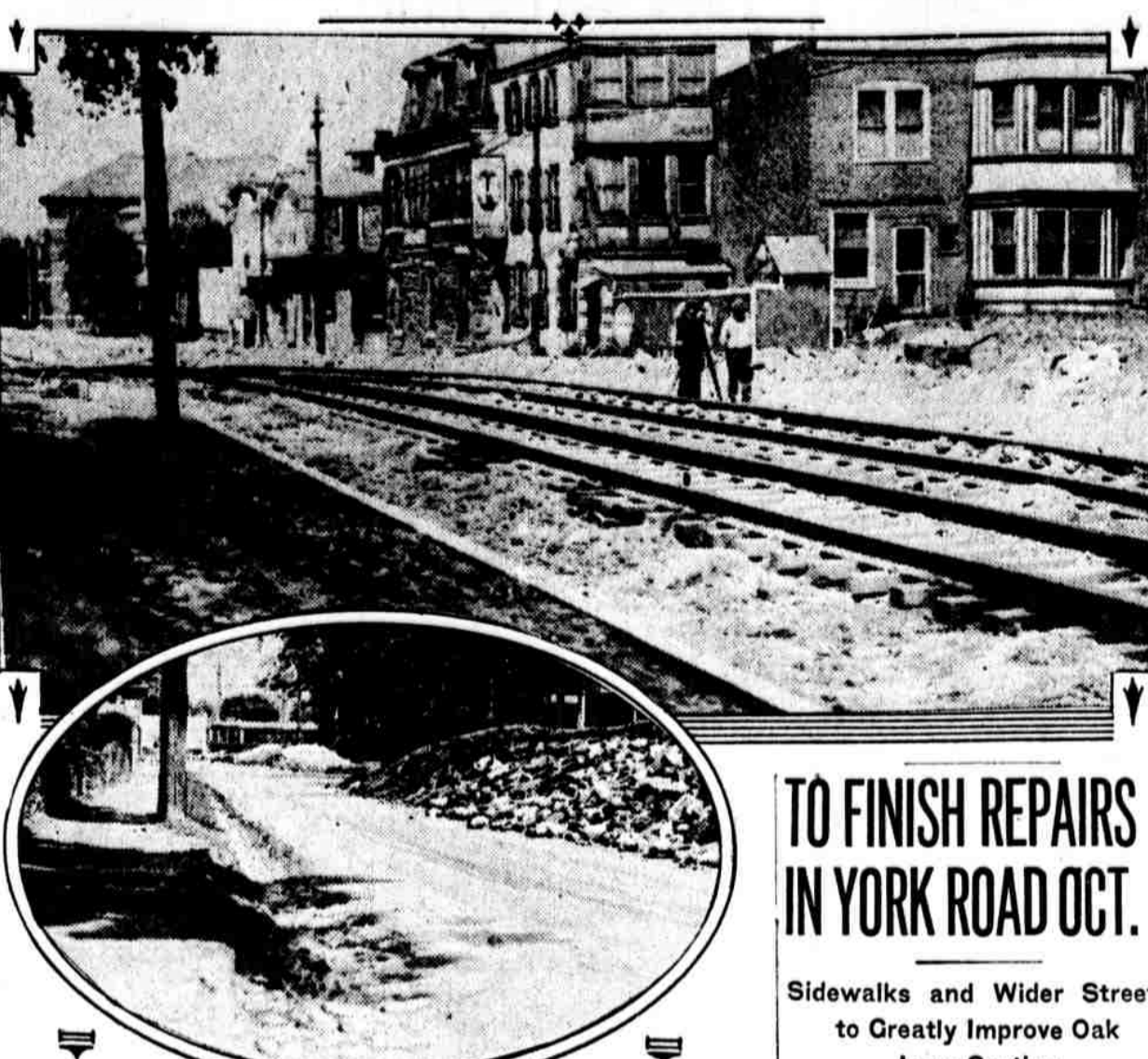
Contractors are at work in the Oak Lane section putting the Old York road in good condition. The upper section shows a bit of Old York road. Below is a section of Spencer street. A sidewalk along Old York road will be one of the most welcomed improvements from Oak Lane to City Line.
